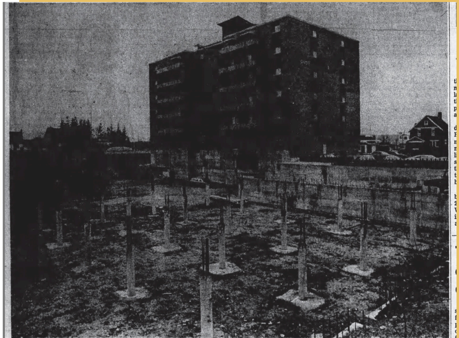
This is all there is to the Lord Kitchener Hotel project at Weber and Dellroy Streets. Money troubles killed it several years ago. Record Photo
